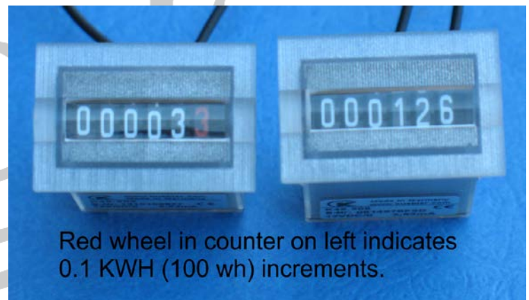
Figure 6. Example of a typical indicator. Any indicator that operates properly with the system is acceptable. The left counter indicates at 3.3 kWh and right counter indicates at 126 kWh.
