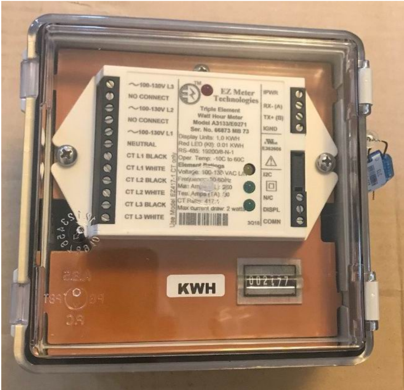
Figure 1. Photo example of the meter ID in a NEMA-enclosure and the Category 1 wire terminal installation sealing provision.
